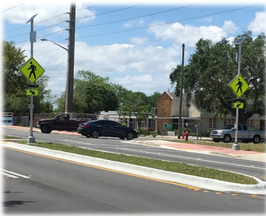
BMSD Safe Streets Project – Phase I : landscaped medians, decorative crosswalks with flashing beacon and bike lanes from NW 24 Ave and 6 Street (Sistrunk Blvd) – pictured-down to 27 Avenue
