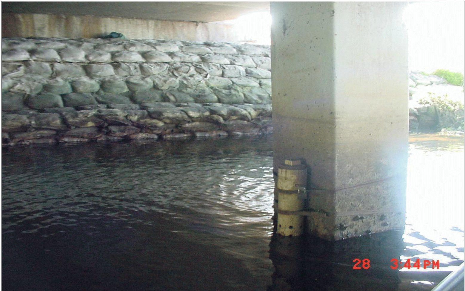
Figure 6. YSI Datasondes Housed and Locked in Perforated PVC Casings Attached to the Bridge Pilings at Martin Luther King Boulevard (Site 101), Sistrunk Boulevard (Site 64), and Broward Boulevard (Site 16). The PVC casing at Site 113 was setup midstream approximately 35 meters north of the CS 17 water control structure (from BCDPEP 2002).
