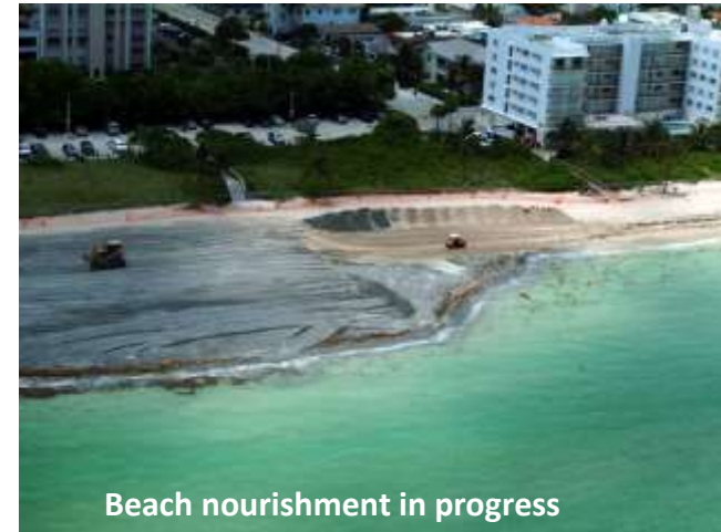
Beach nourishment in progress Recent projects have nourished 4.6 miles of shoreline and constructed 1.5 miles of dunes.
