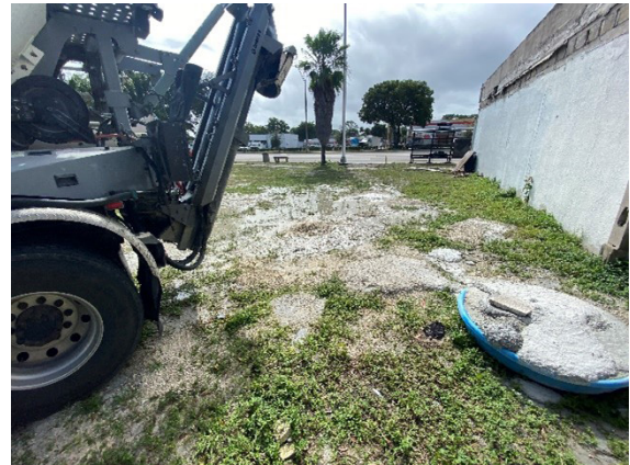
Cement truck chute being washed onto bare ground of vacant lot.
