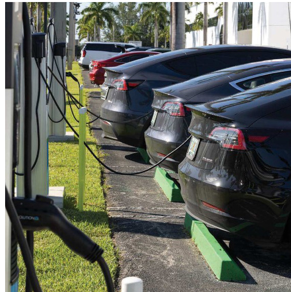
19 Electric Vehicle Charging Stations at three Showrooms Including twelve installed at CITY Furniture Corporate Headquarters
