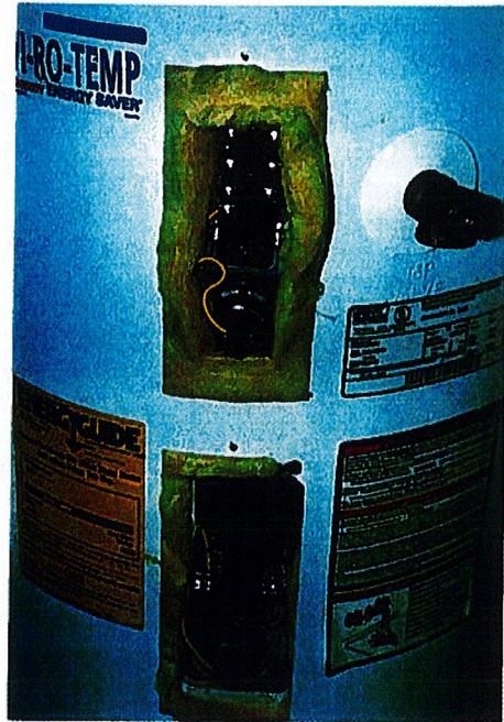
PHOTO 1—"Low boy" electric water heater with side covers removed showing thermostats, wiring and heating element connections.
