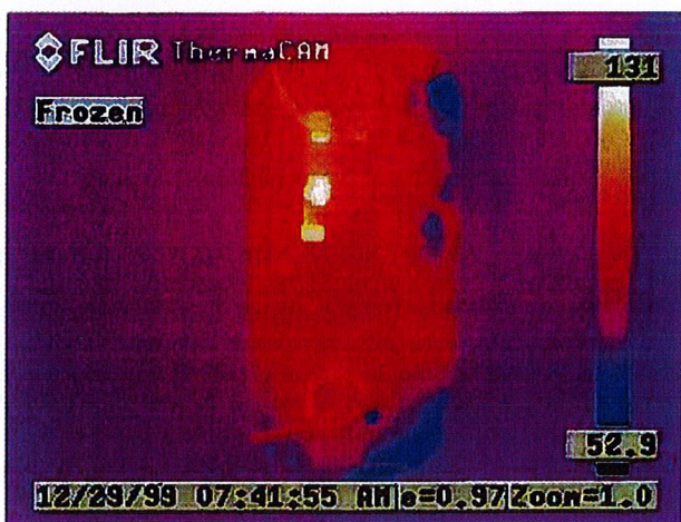
PHOTO 5—This thermal image shows the results of loosened connections on the thermostat and high limit switch of an electric water heater.
