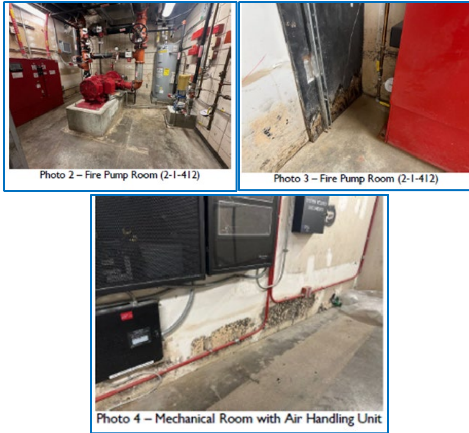
Figure 34 Images from the December 12 th Survey Report Showing Water Damage in the Fire Pump Room and Mechanical Room
