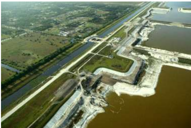
L-8 Reservoir Modifications Pump Station and Inflow Structure
