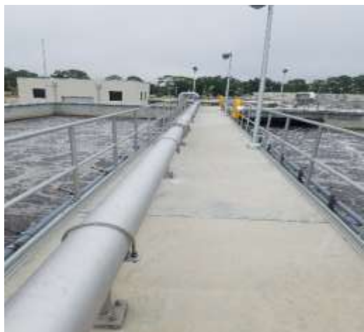
A new anoxic basin, aeration basin, and air and process piping was constructed to expand the MLE
