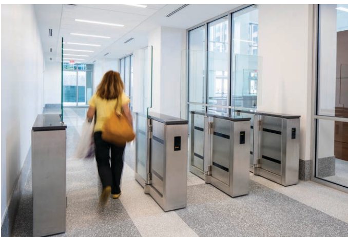
Employee security access point, Broward County Judicial Complex
