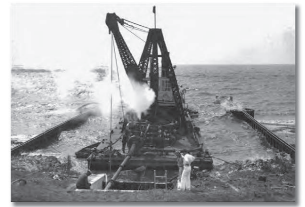
Floating crane working on the Central and Southern Florida Project at Lake Okeechobee.
